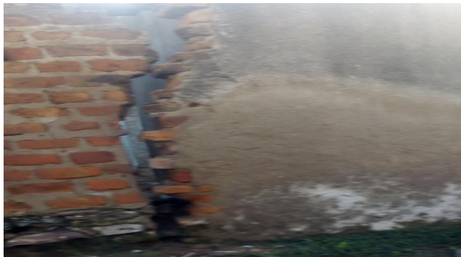
Figure 17.1 Cracks and collapse in buildings
